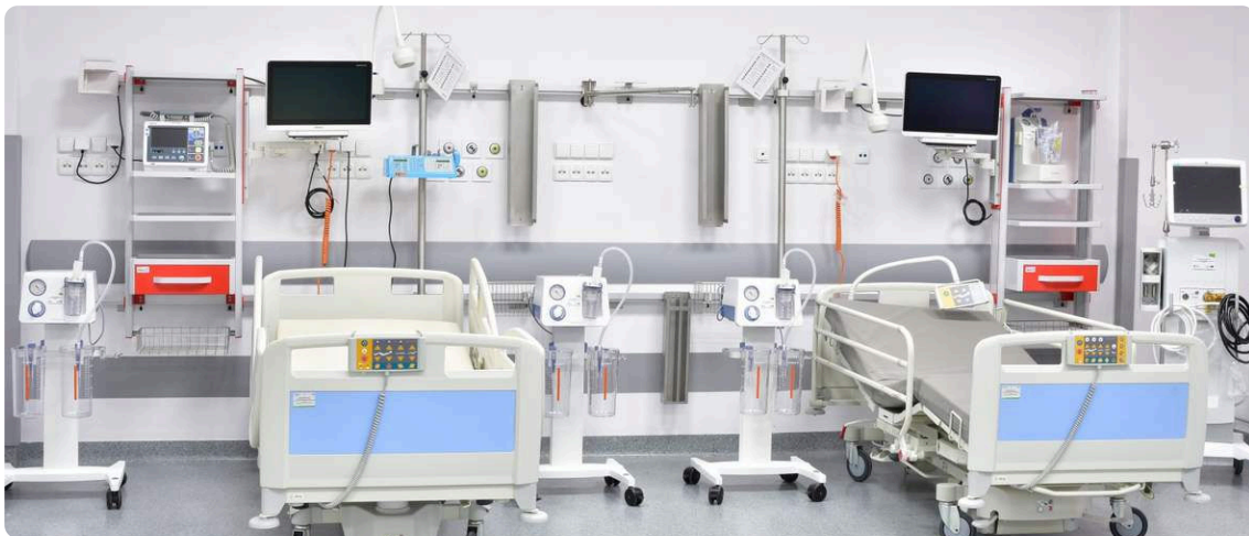
Bed bay with ISA rail. Intensive care unit at the university hospital in Bydgoszcz: one continuous wall rail per bed bay carries monitor, flowmeter, shelves and disposal and keeps cables and equipment off the floor.
